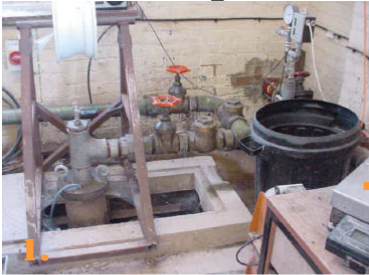
1. Water is pumped from a 60 metre bore hole at a rate of 50m 3 /hour
