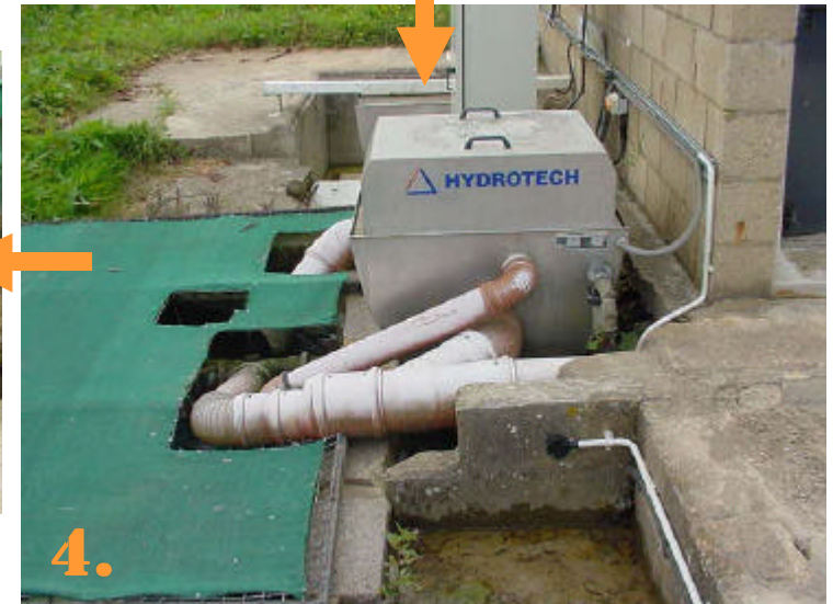
4. Water is passed through a filtration system before being pumped to the second header tank for re-use.
