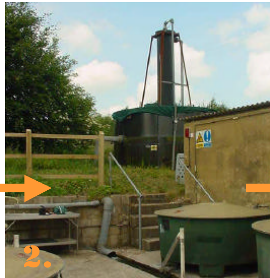
2. Water is pumped to the header tank where it is degassed.
